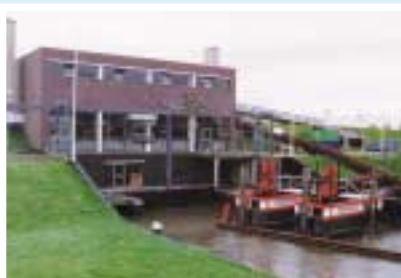
Several emergency pumps have supported Boezememaal Westland since early 2000. During the storms of November 2000, they prevented worse things from happening. In 2001, the capacity of the pumping station was tripled permanently.
